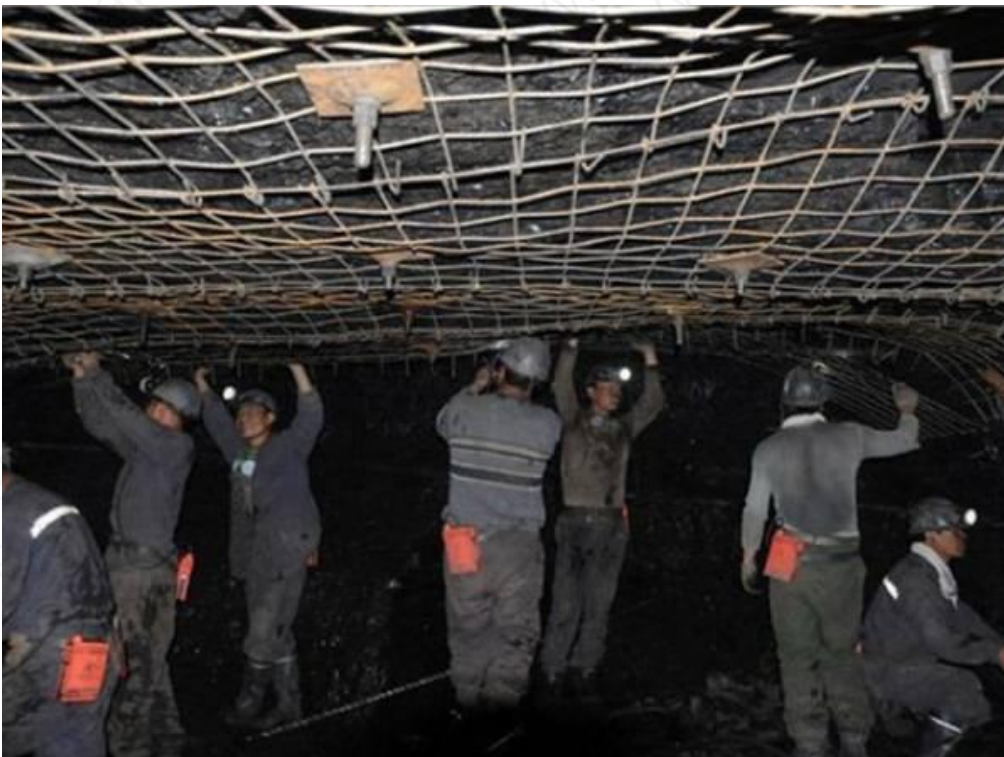
For Diamond Mining Under Ground Support Mesh
