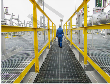
Steel grating platform walkways
