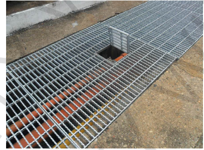
Steel grating trench covers
