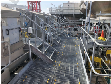
Steel grating platform mezzanine
