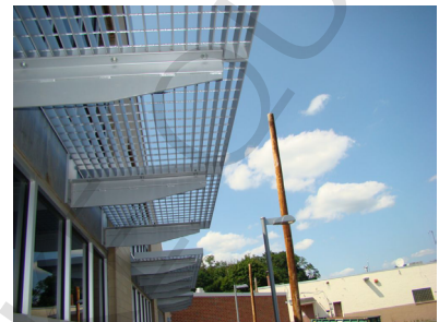
Steel grating sun shade panels
